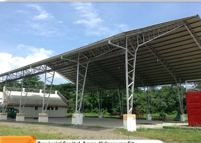
Provincial Capitol, Amas, Kidapawan City Construction of the Multi-Purpose Covered Court Phase II 6m x 14.4 m MP Building with Toilet and Bath. Food Court and Bleachers Project Cost: 1,855,885.40
