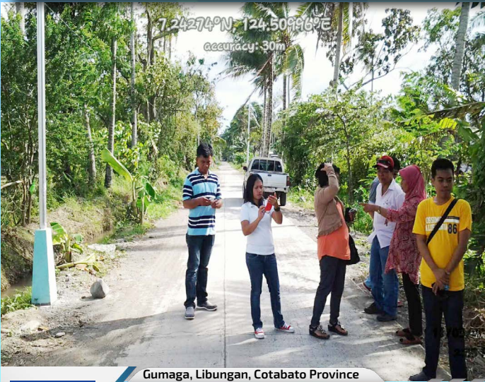
Project Cost: 1,048,727.25 Gumaga, Libungan, Cotabato Province Improvement of Katitisan-Gumaga FMR Road concreting with length: 300 Width: 7 meters with pavement with 5 meters Thickness: 0.15
