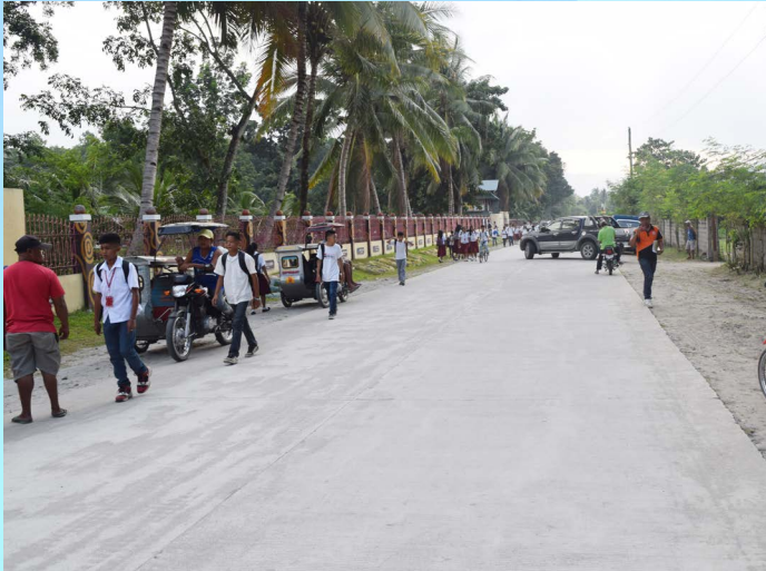
Poblacion, Norala, South Cotabato Project Cost: 2,000,000.00 Concreting of Roads Concrete paving of road with thickness of 0.20 meters, and with total length of 250.00 meters
