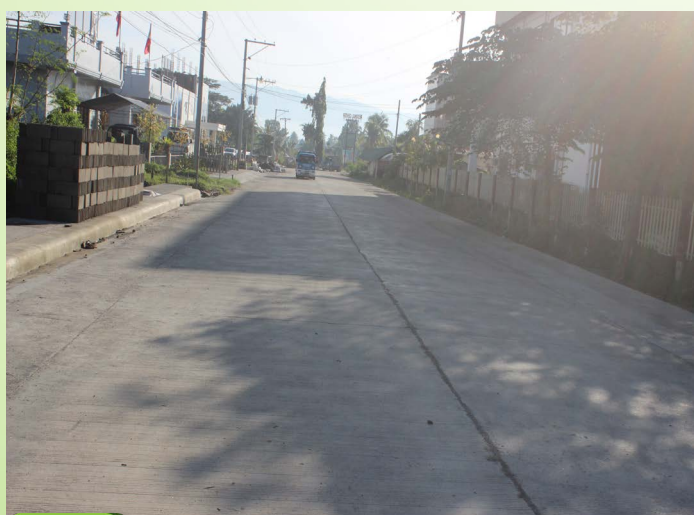
Regional Center, Carpenter Hill, Koronadal City, South Cotabato Project Cost: 7,000,000.00 Concreting of Road with Lined Canal concreting of .015x6.00x223.20 LN.M. road curb and gutter - 122.50 LN.M. lined canal with catch basin - 100 LN.M. gouted riprap (slope protection) - 94.80 CU.M. box culvert (6 units) - 1.00Mx1.30M x 6.00 M
