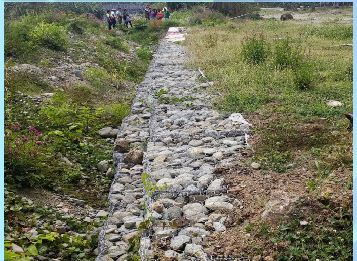
Project Cost: 2,500,000.00 Poblacion, Palimbang, Sultan Kudarat Flood Control and Rehabilitation of Palimbang Bridge Approach both sides Filing Gable Gall filled of Stones
