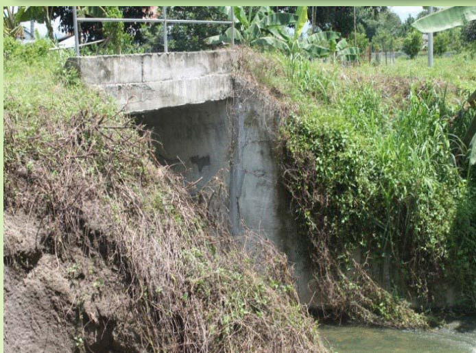
Brgy. Liwanay, Banga, South Cotabato Project Cost: 1,000,000.00 Construction of Concrete Box Culvert with Wing Walls 3m x 3m x 7m RCBC Reinforced Concrete Box Culvert with Wing Walls and Aprons
