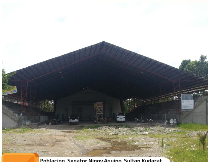
Project Cost: 2,211,893.00 Poblacion, Senator Ninoy Aquino, Sultan Kudarat Improvement of Municipal Gymnasium Construction of Bleacher with steel truss and roofing including the repair of CR & Fabrication of Window Grills
