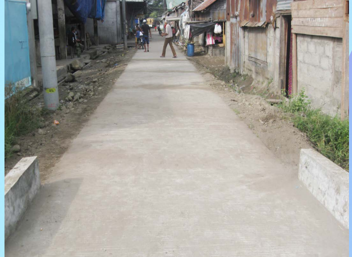
Project Cost: 1,006,747.81 Public Market, Lambayong, Sultan Kudarat Concreting of Public Market Alley Composed of Concrete Pavement and Embankment
