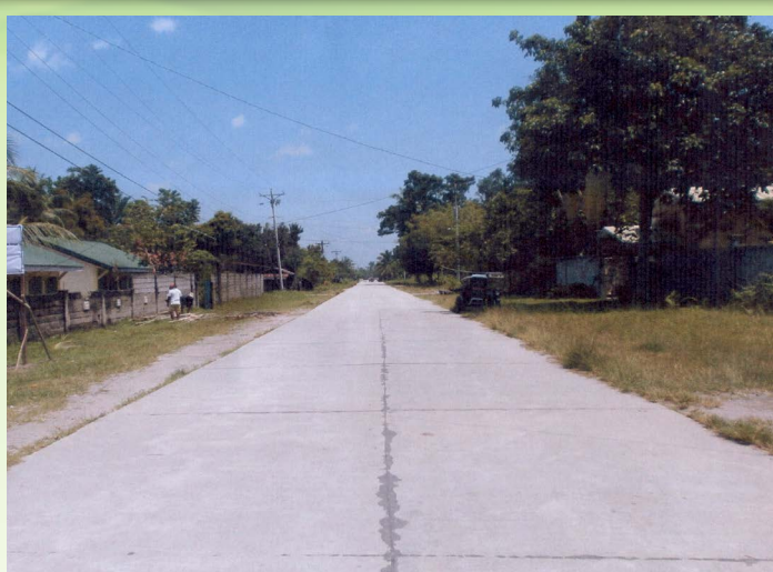
Brgy. Poblacion, Norala, South Cotabato Project Cost: 2,000,000.00 Additional Concreting of Roads at Manuel L. Quezon Street Length: 270 Ln.m. Thickness of PCCP: 0.15 m. Item 200: 0.15 m Item 200: 0.15 m. Item 201: 0.20 m. and PCCP: 6.0 m
