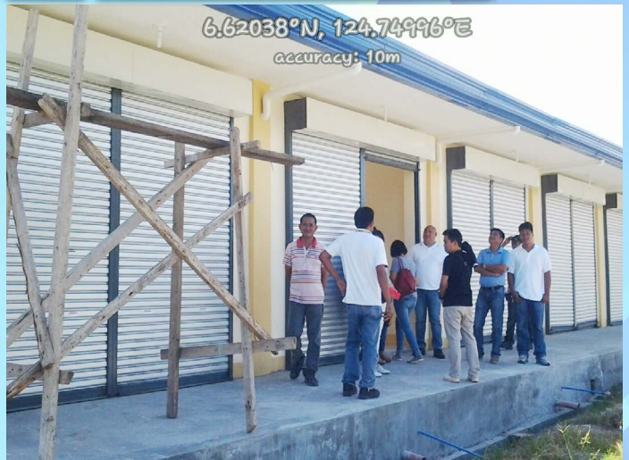
Public Market, Tantaran, South Cotabato Project Cost: 2,000,000.00 Construction of Market Stalls Construction of Additional Six (6) Market Stalls with Ceiling, Electricals and Painting
