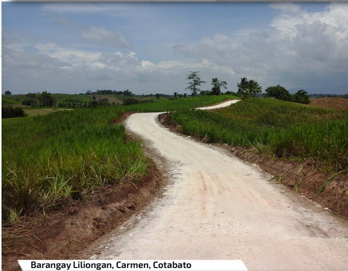
Barangay Lilionan, Carmen, Cotabato Rehabilitation of Road from Crossing Mainline to Sitio Mikalyawa 1,800 kilometer rehabilitation/repair of Farm-to-Market Road
