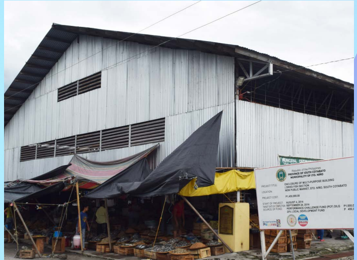
Public Market, Sto. Niño, South Cotabato Project Cost: 1,000,000.00 Enclosure of Multi-Purpose Building Installation of roll-up doors
