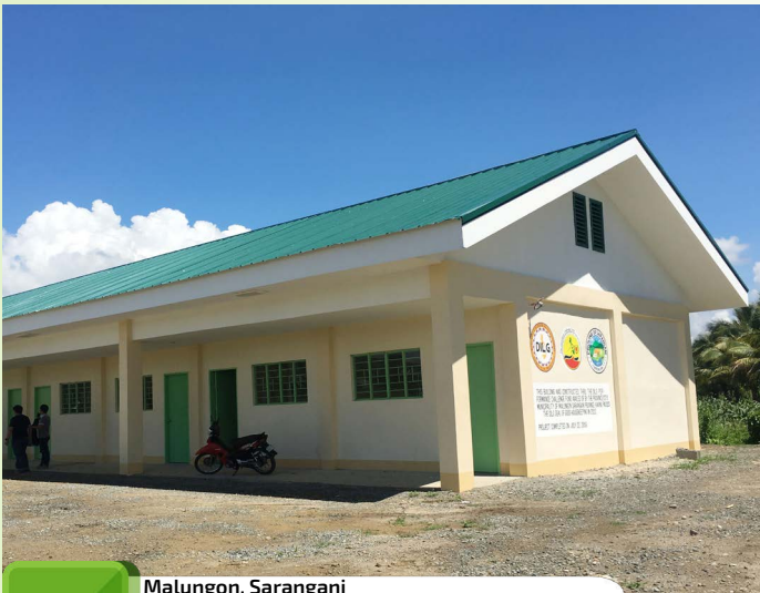
Malungon, Sarangani Construction of School Building Mindanao State University Extension Project Cost: 6,000,000.00
