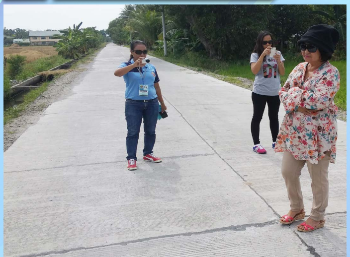
Grino and Ledesma, Tacurong City, Sultan Kudarat Project Cost: 3,000,000.00 Concreting of Brgy. Road connecting Brgy. Grino and Ledesma Concrete paving of road with a pavement width of 5.0 meters, thickness of 0.20 meters, and with total length of 250.00 meters
