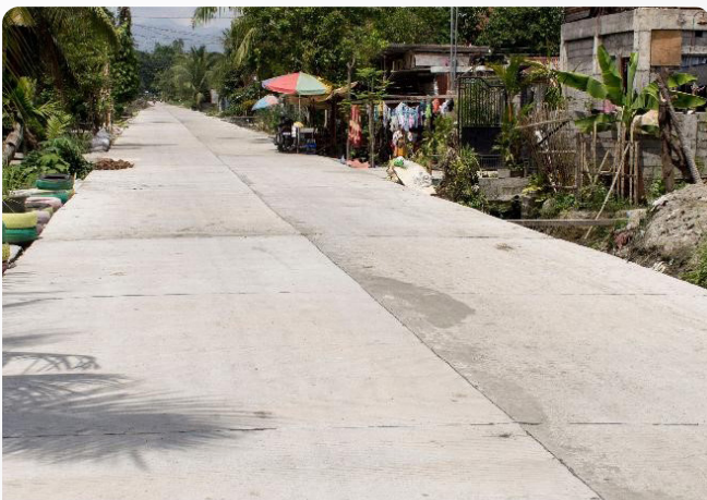
The concreted Bougainvilla to Junction Orchid Street worth Php 2.3 million in Barangay Libertad, Surallah, South Cotabato provides better road access to residents and commuters.
